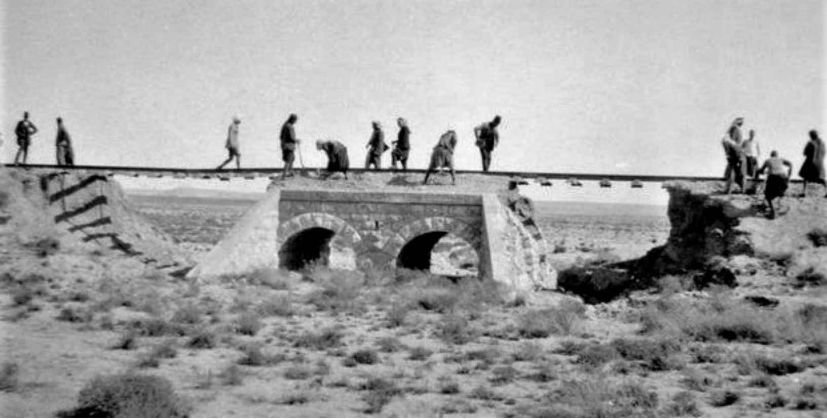
Repairing the railway track near Maan, 1918 – Author, T. E. Lawrence, Imperial War Museums, public domain, Wikimedia
